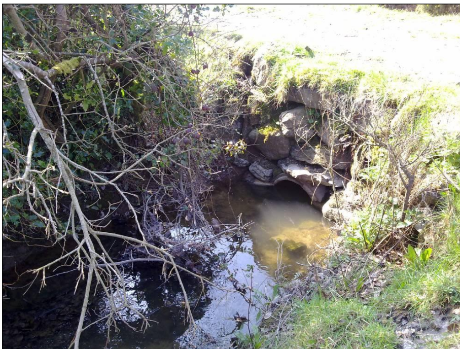
Photograph 25 – Typical Culvert along the Aggard Stream which requires replacement
