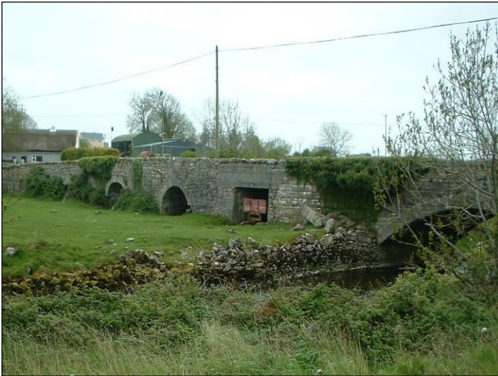
Photograph No. 10 Upstream face of the Dunkellin Bridge showing the main arch and flood eyes on the left bank
